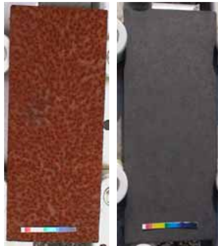
Fig.6 Surface appearance of non-coated (left) and coated (right) steels, after 2 years Corrosion. Air-borne salt content was 1.0 mdd.
